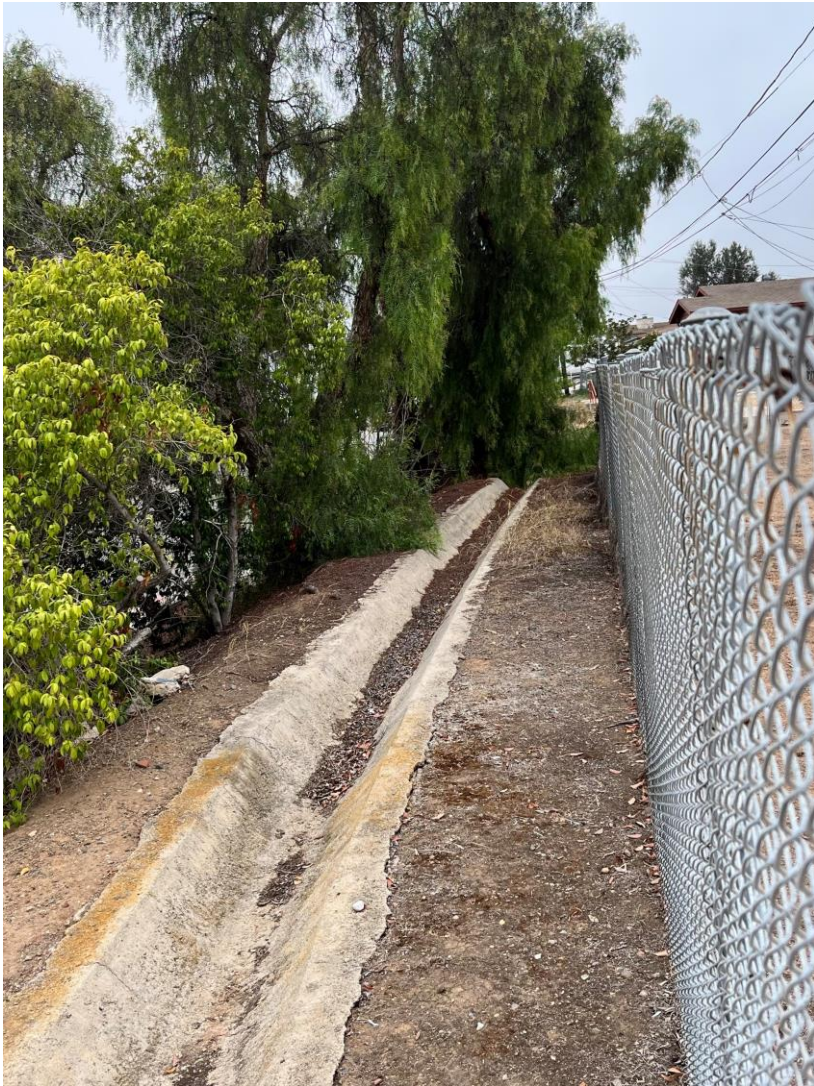
Brow ditch east of Orange Street cul-de-sac
