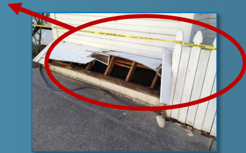
Cripple wall collapse
